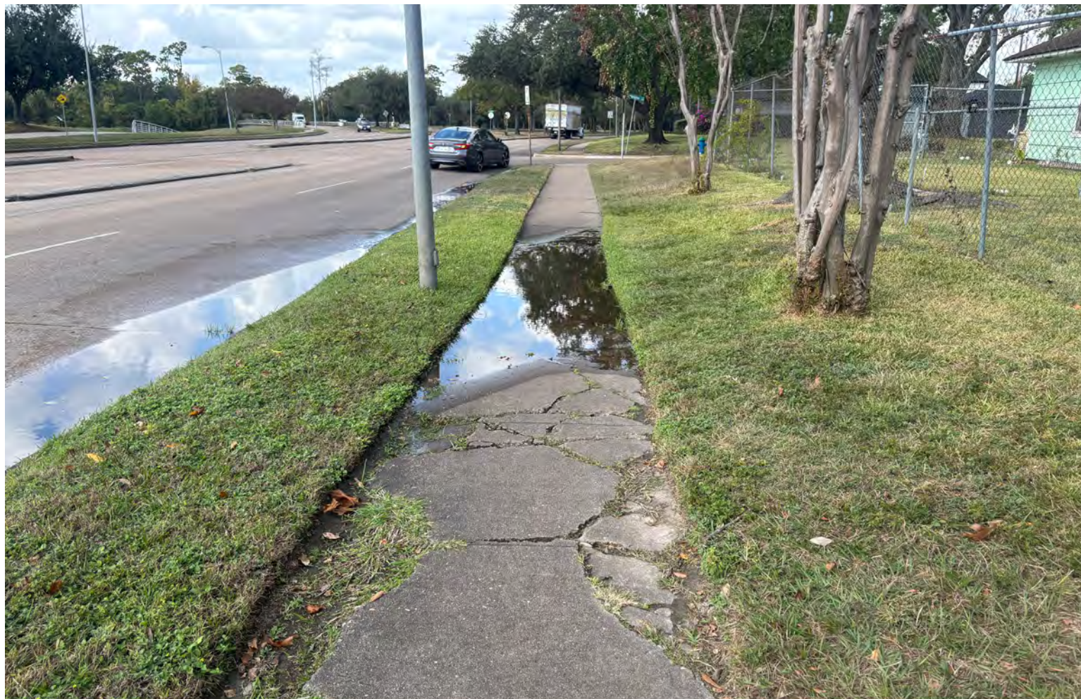
Broken sidewalks with drainage conflicts, TC Jester Blvd
