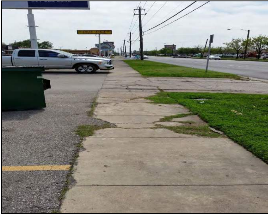
Photo 13 – Sidewalk cracking and grass growing between the cracks at Shepherd Drive
