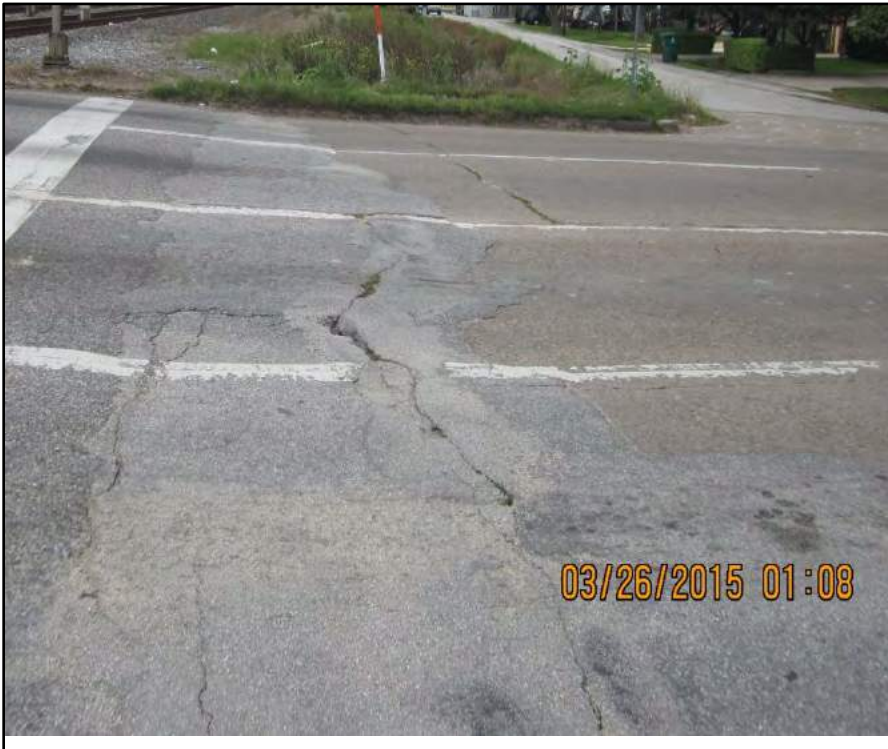
Photo 8 – Cracks through patches
