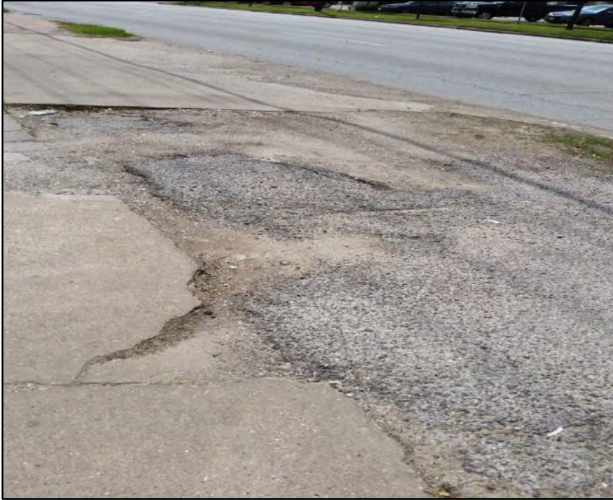
Photo 3 – Settled sidewalk, uneven and weathered patching
