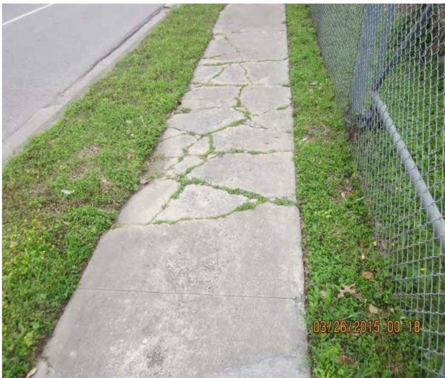
Photo 12 – Cracked sidewalk in Shepherd Drive
