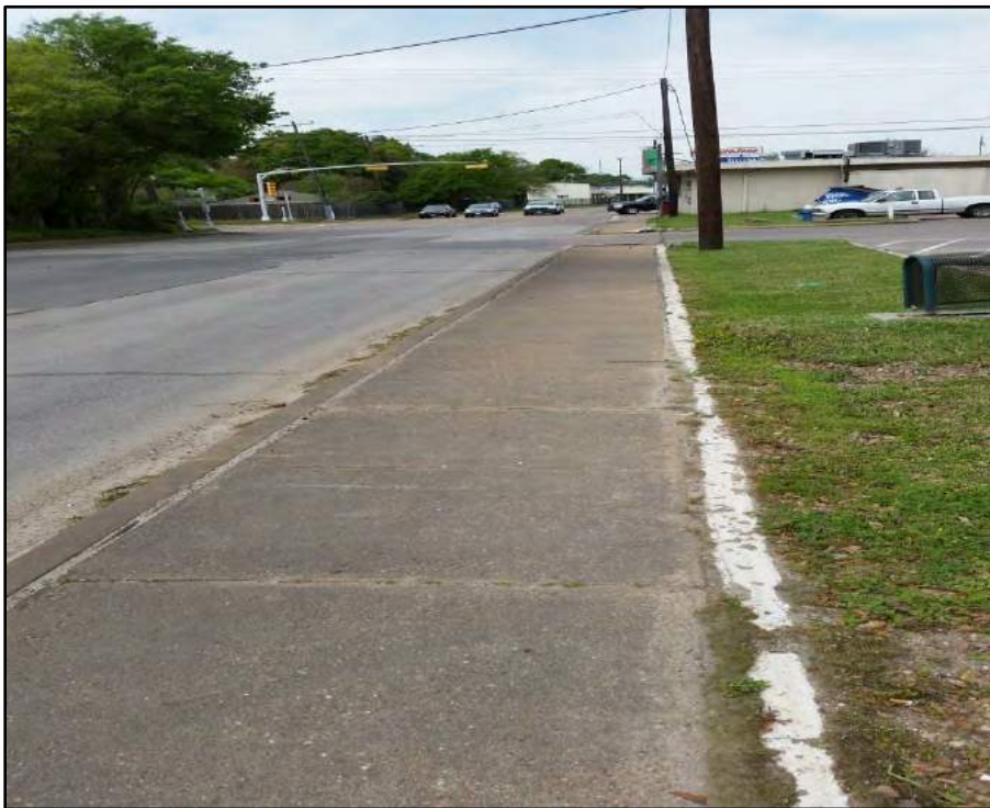
Photo 10 – Crack at ends of sidewalks on Durham Drive
