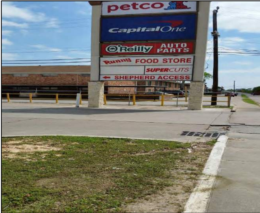
Photo 11 – Settling drain along Durham Drive
